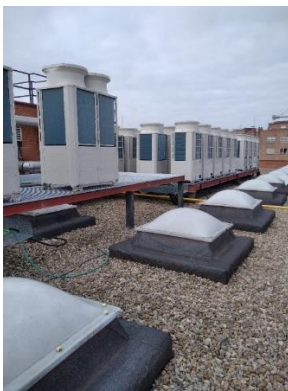
New heat pumps (aerothermal)
