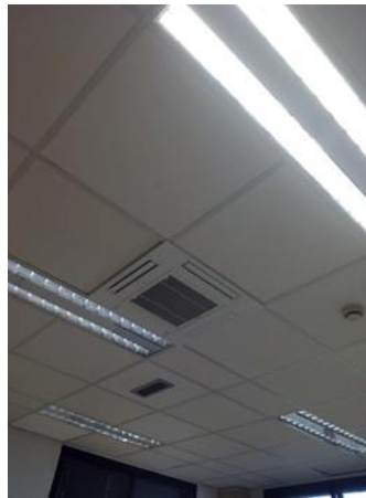
New indoor units
