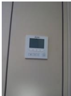
New individual control systems
